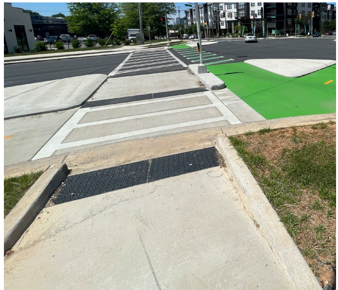
A curb ramp should provide tactile warning strips and a slope that supports users with vision and mobility impairments.
